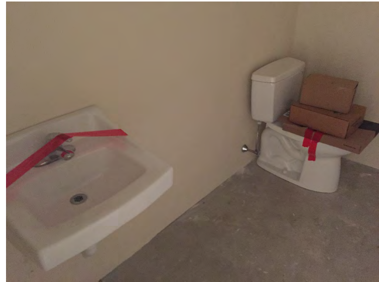
View of bathroom appliances
