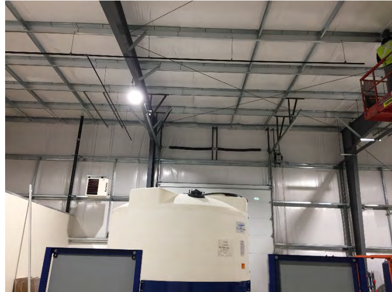
View of overhead propane lines for heaters
