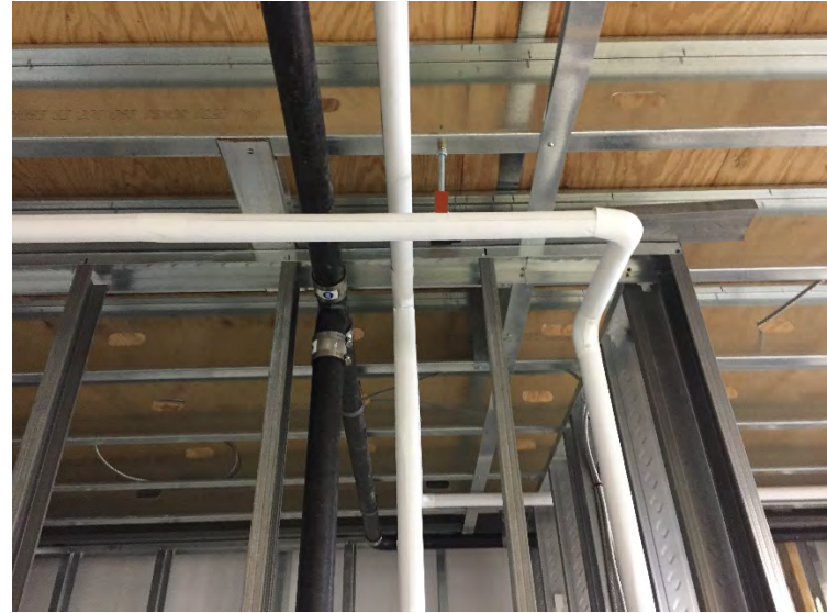
View plumbing in office
