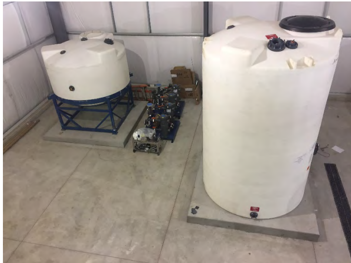
View of treatment system components
