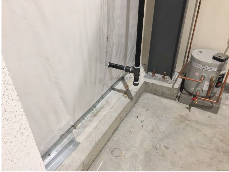
View of propane line exiting building
