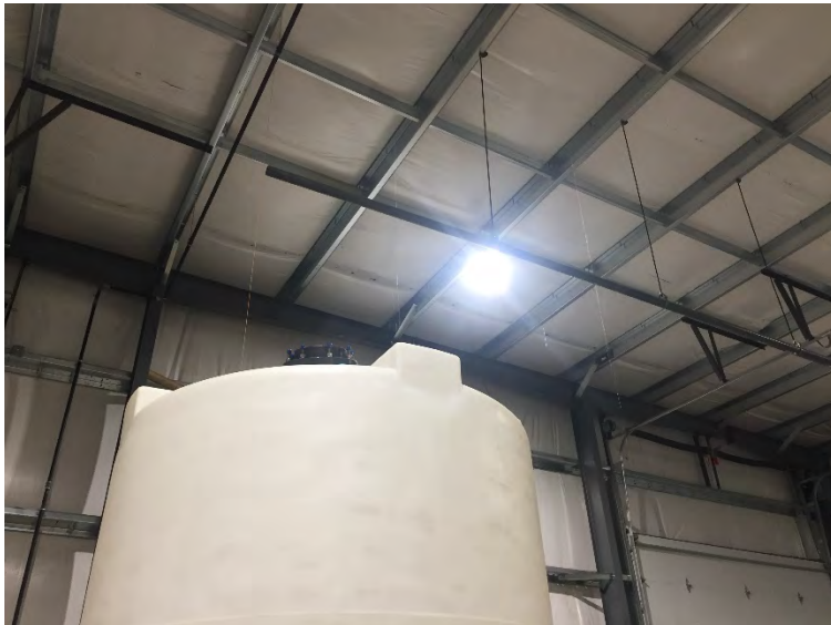
View of building roof leaking
