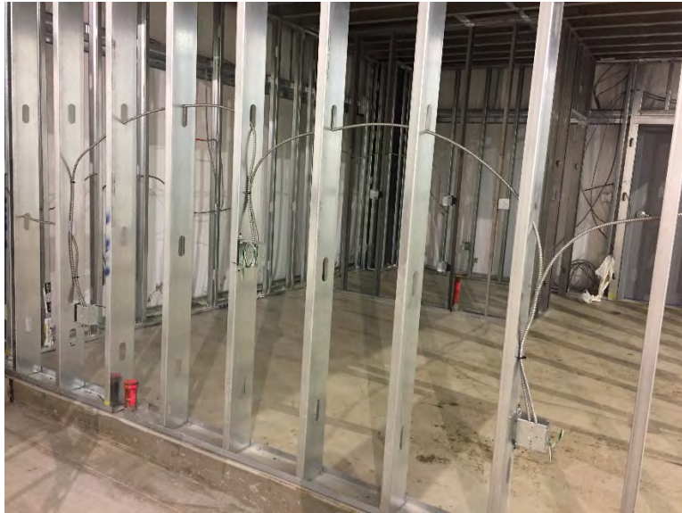
View of preliminary office electrical
