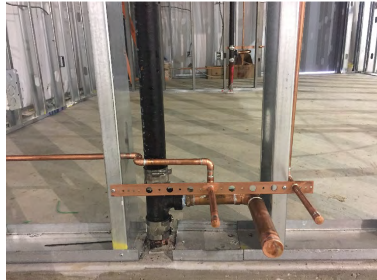
View plumbing in office
