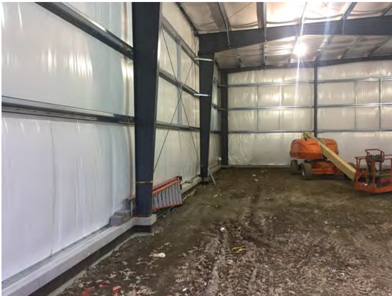
View temporary indoor lighting
