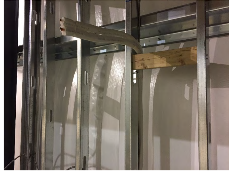
View of AC piping in office
