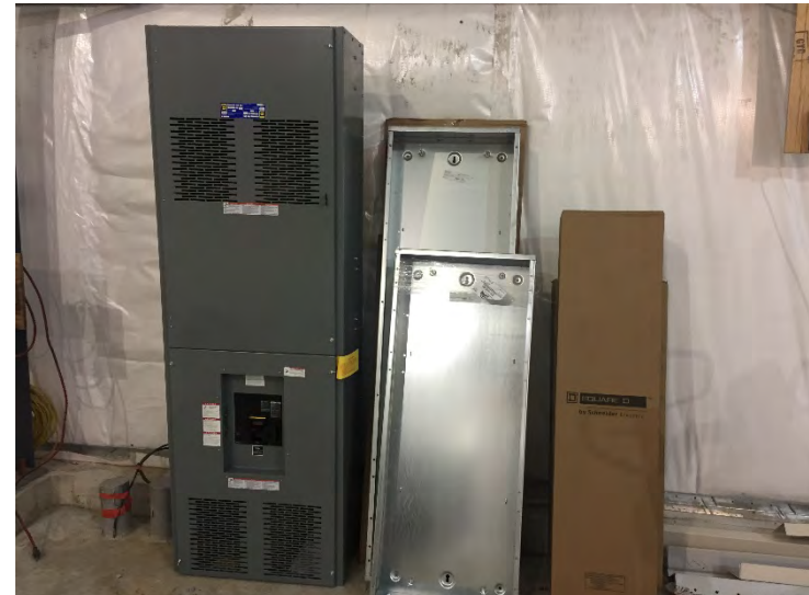
View of system switch gear panel
