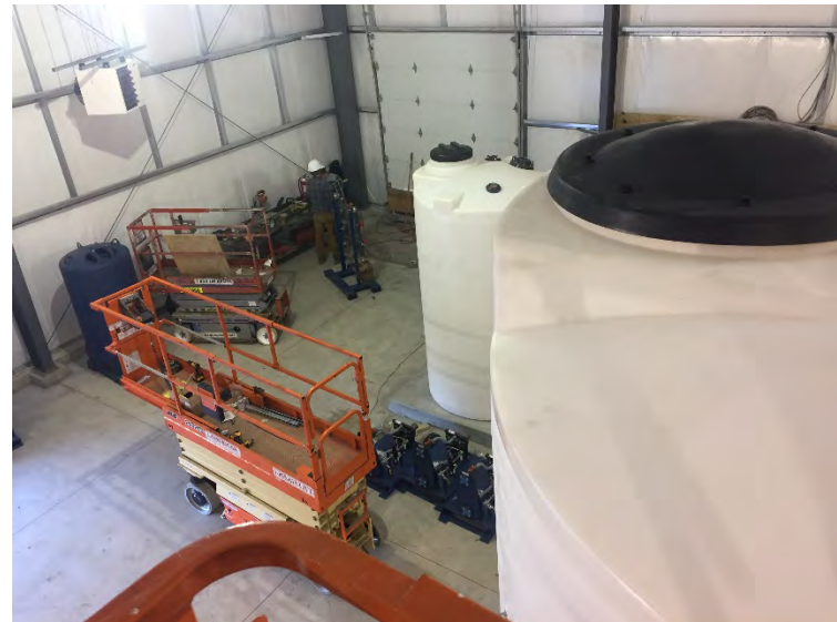
View of treatment system components
