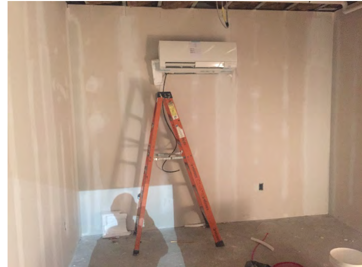
View of office air conditioner
