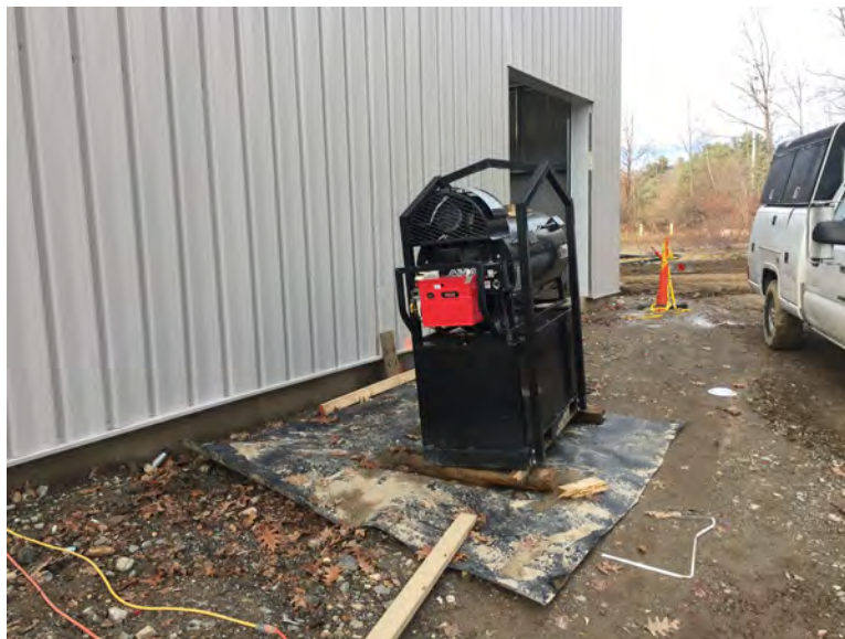
View of diesel heater to temporarily heat the interior of the building
