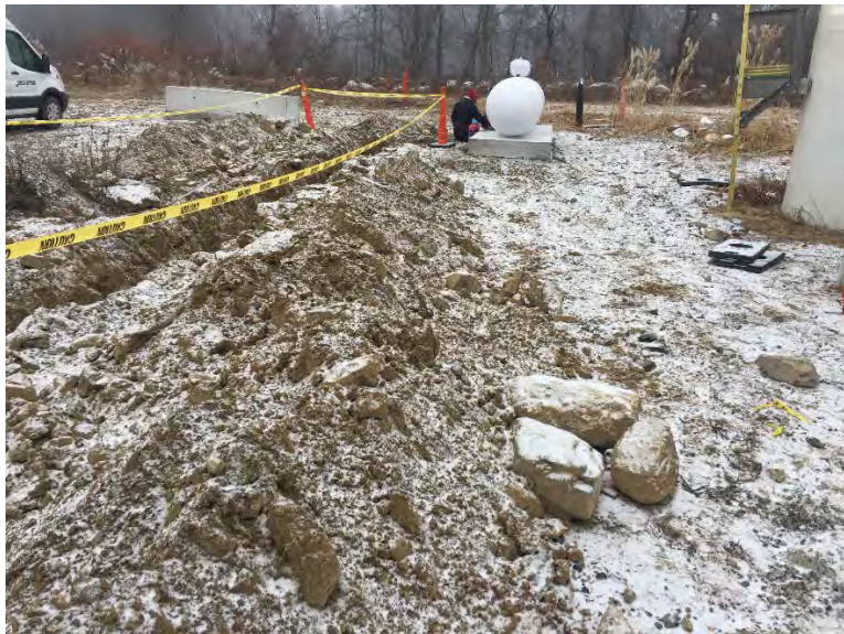
View Propane Tank
