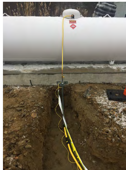
View Propane Tank
