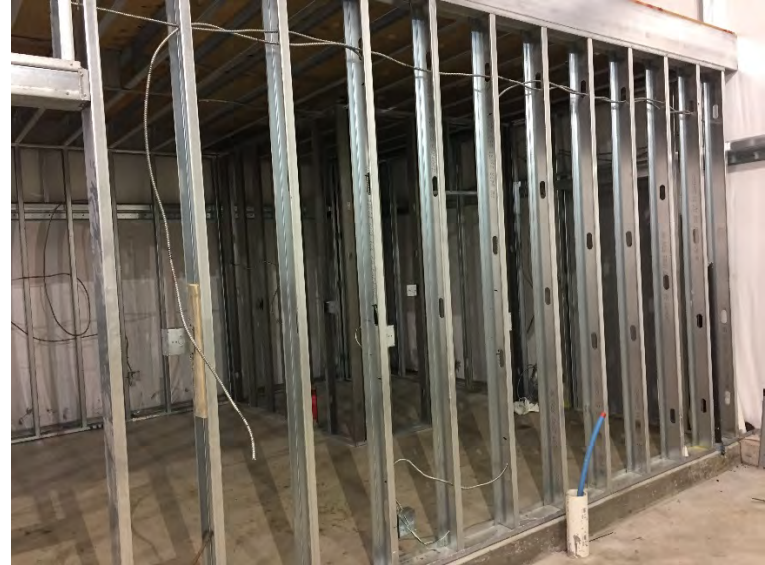
View of preliminary office electrical
