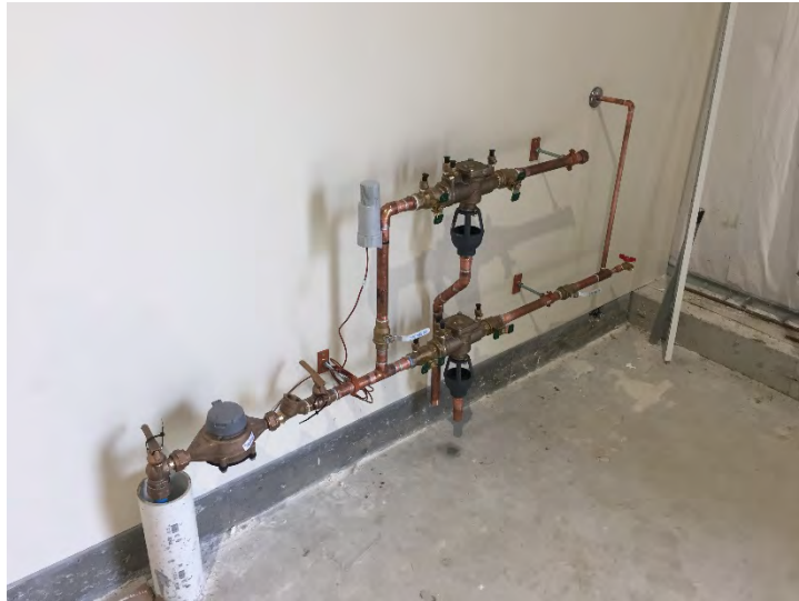
View of water entrance and water meter
