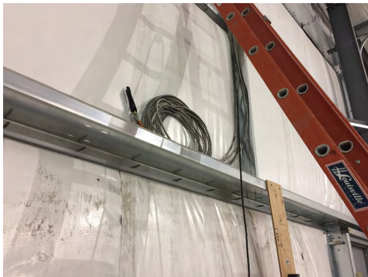
View of electrical work in building
