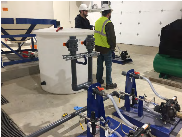
View of pump branch and AECOM rep.
