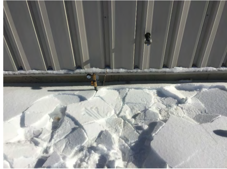
View of ground and building propane stubs
