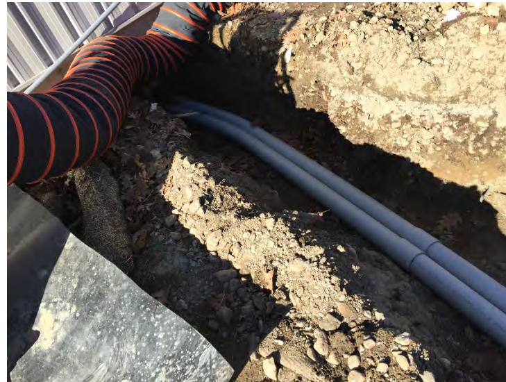
View electric line from building to pole
