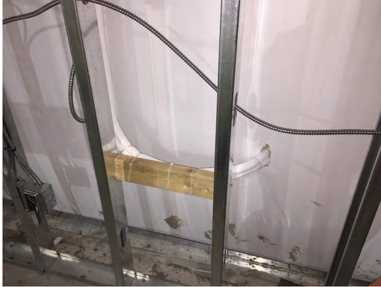
View of AC piping in office
