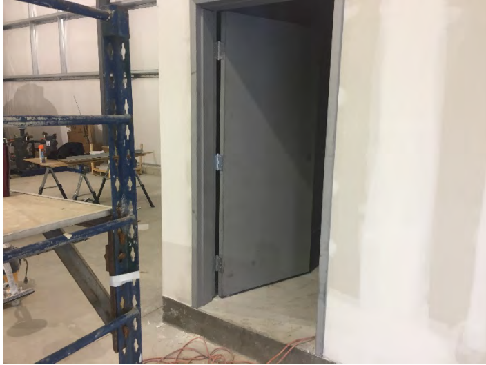
View of installed office doors
