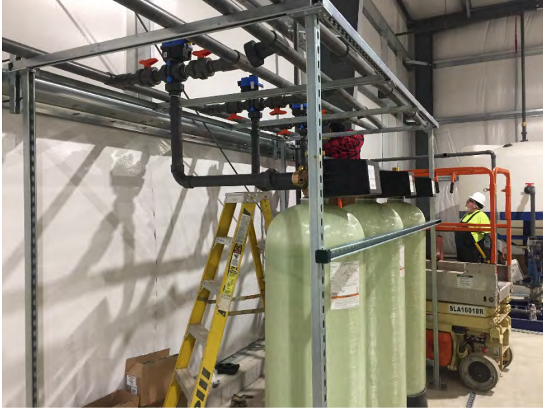
View TPC Multimedia Filters and Tree system
