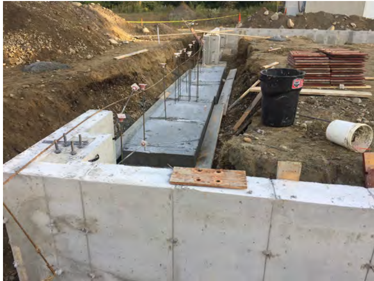
Settled concrete from day before
