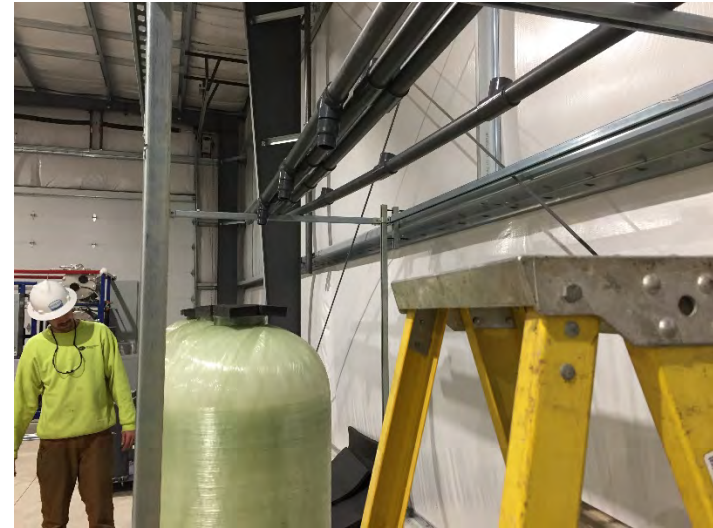
View of multimedia filters and piping frame
