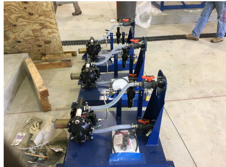
View of treatment system equipment in building
