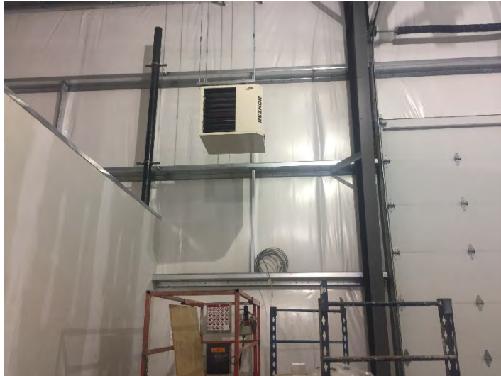
View of building heaters
