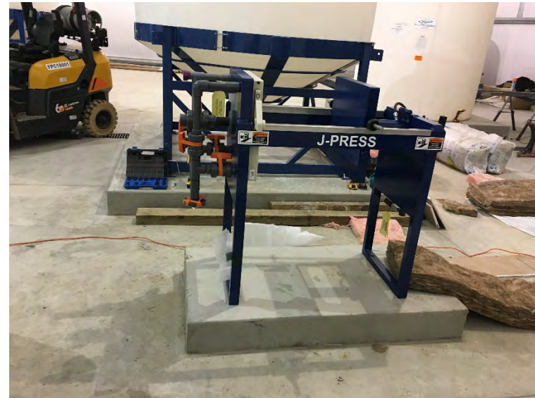
View of treatment system equipment in building
