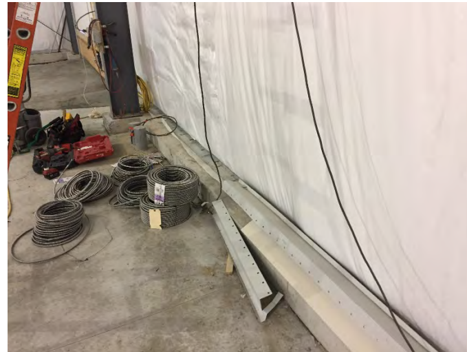
View of electrical work in building
