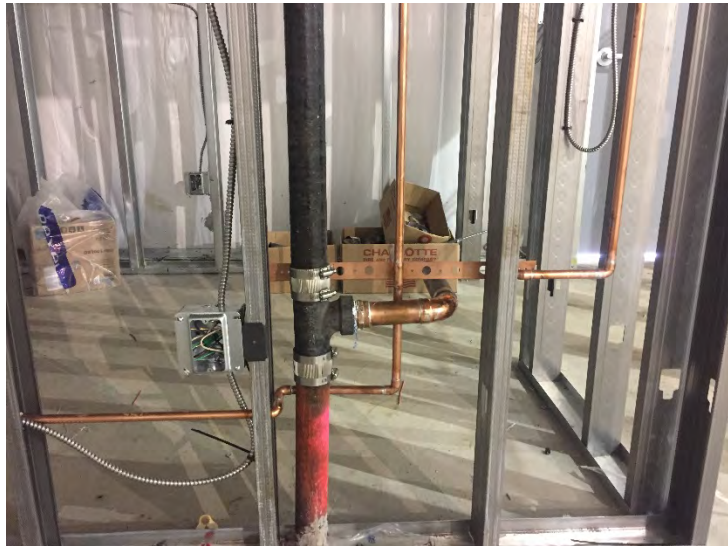
View plumbing in office
