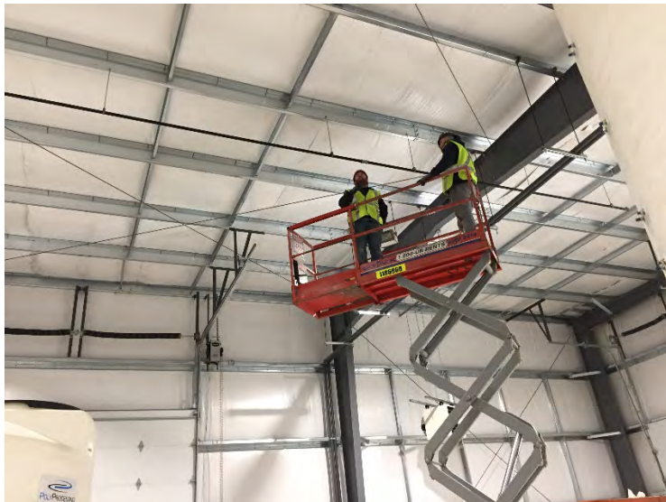
View of overhead propane lines for heaters
