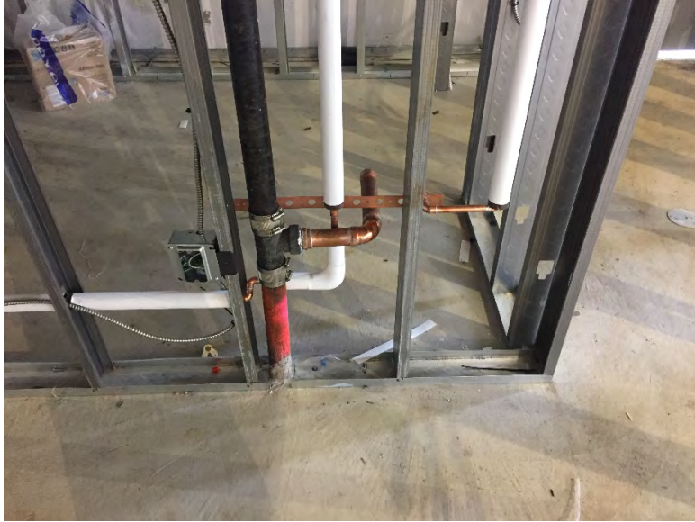
View of plumbing insulation
