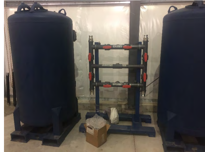
View of treatment system parts
