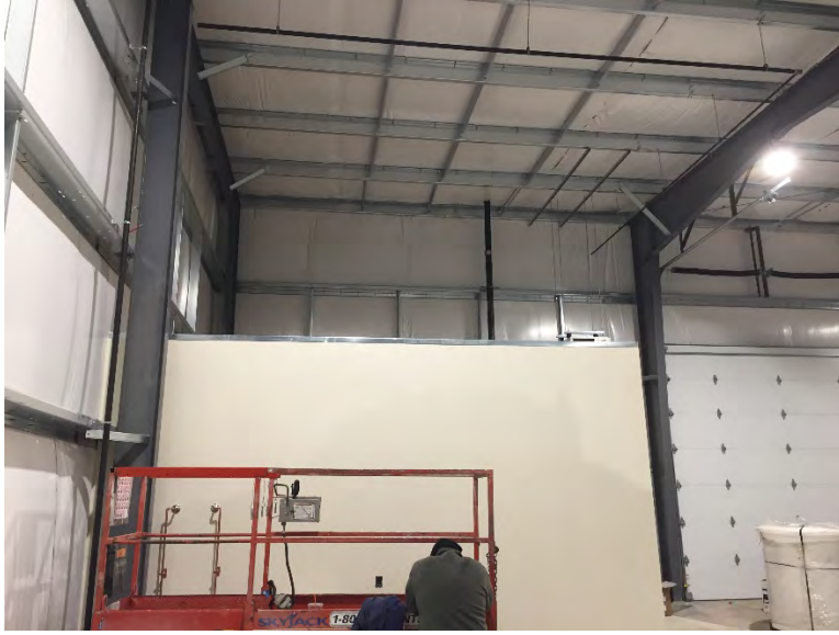
View of overhead propane lines for heaters
