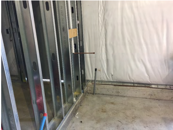
View plumbing outside of office
