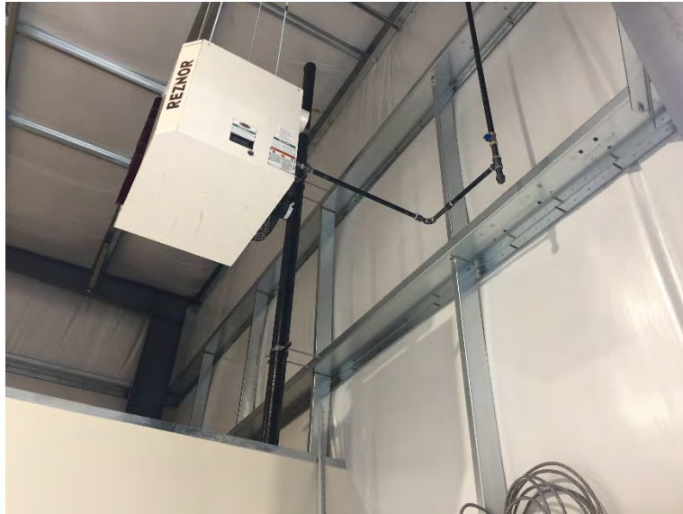
View of overhead propane lines to heater
