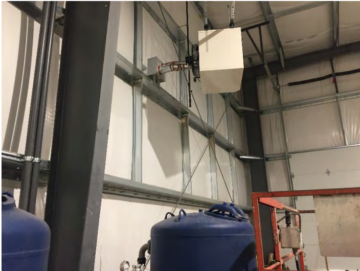
View of heaters and vents
