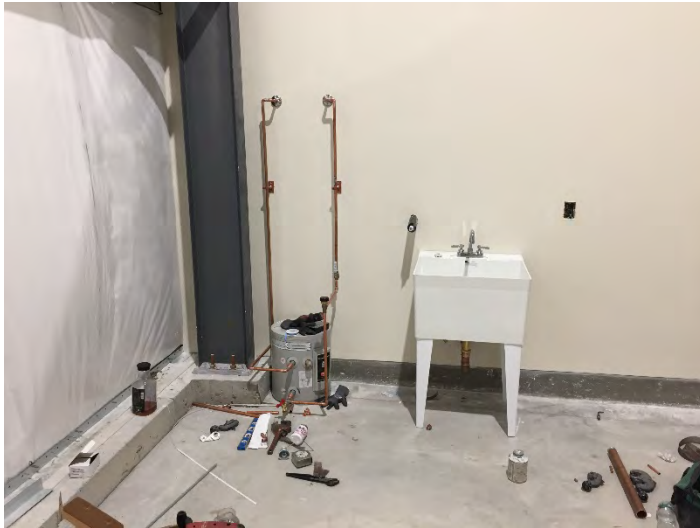
View of slop sink, and hot water heater
