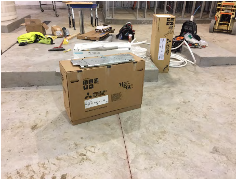
View of AC in box
