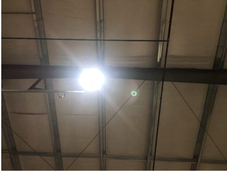
View of building roof leaking
