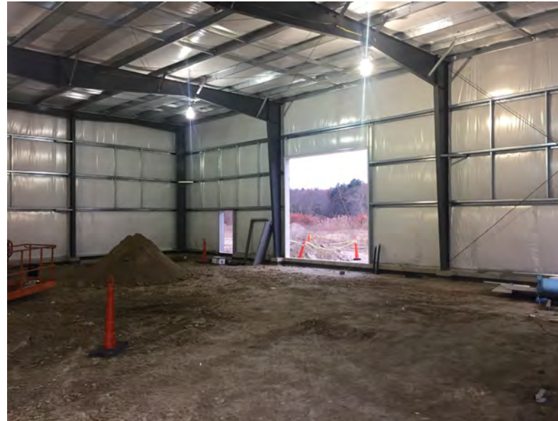
View temporary indoor lighting
