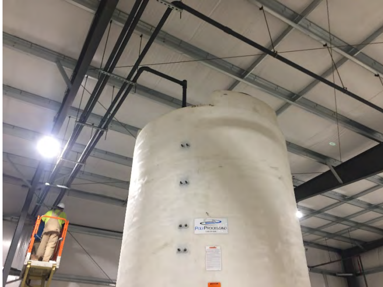
View of system overhead piping to tank
