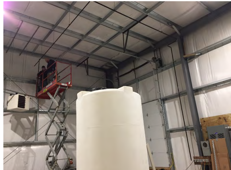
View of overhead propane lines for heaters
