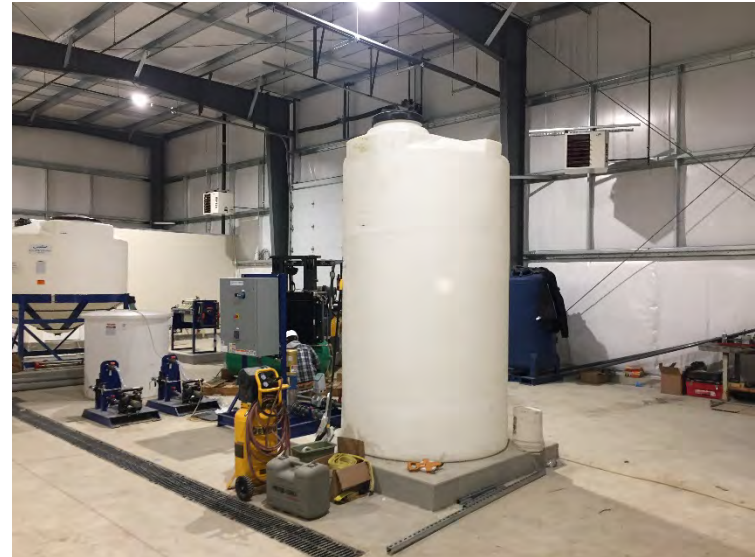
View of system components and overhead gas/water lines
