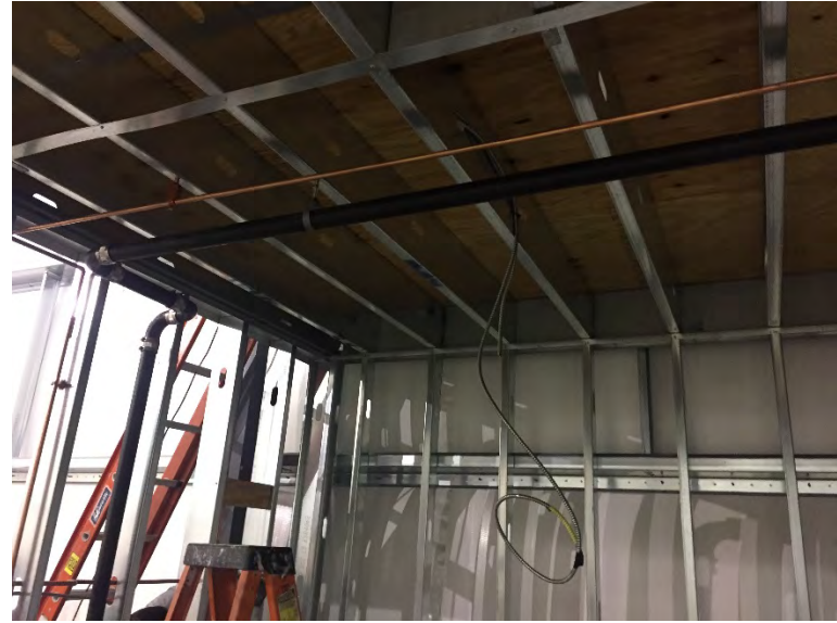
View plumbing in office
