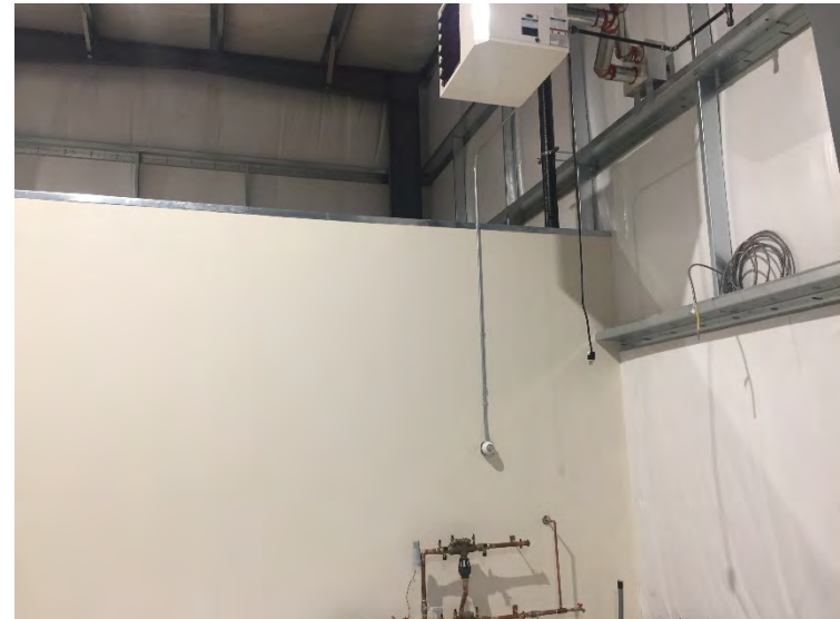
View of heater controls installed on Tuesday
