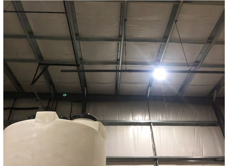
View of building roof leaking
