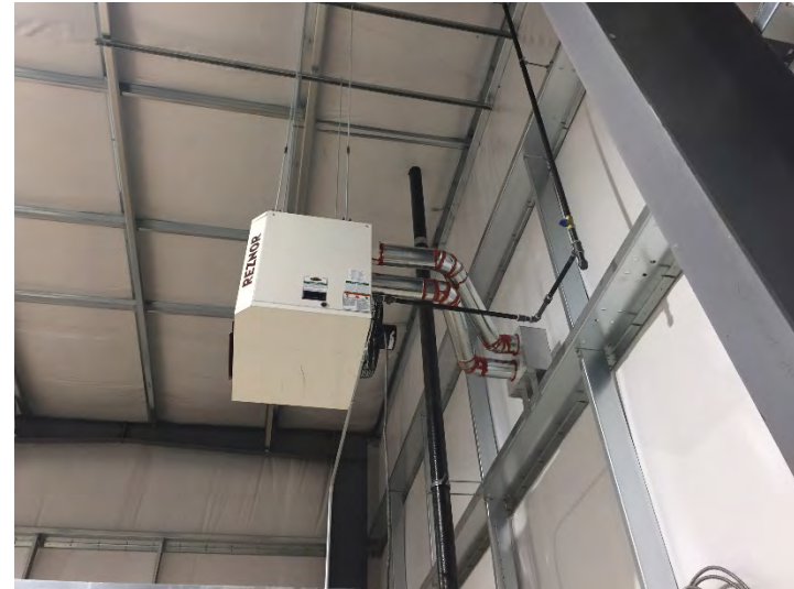
View of heaters and vents
